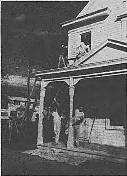
Finisse Co. painters are giving the Old Hicksville Courthouse at Heltz Place a fine face-lifting these days. The National Historic Building, the home of the Gregory Museum, has been the object of a Town of Oyster Bay Community Development/Preservation Project since the summer.
