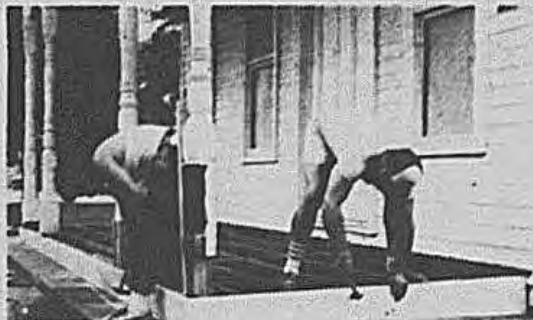
Workmen of Unicorn Contractors are shown replacing the original front porch at the Old-Heltz Place Courthouse. The Gregory Museum Historical Committee has worked with the Town of Oyster Bay's contract architects, Weiderscham Associates, in trying to assure the authenticity of appearance in preservation and restoration work at the National Historic Building.
