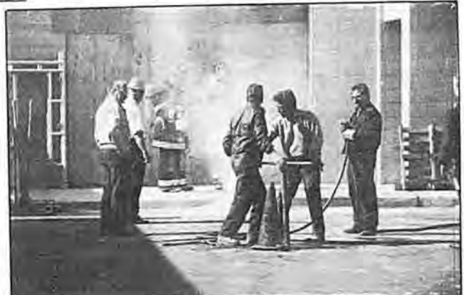
LILCO crewmen attempt to shut off the gas while Hicksville Fire Department Haz-Mat Richard Russell and Brian Kohn (in rear) monitor the immediate area around the leak for pockets of natural gas which in some cases could be ignited by a flick of a light switch.
