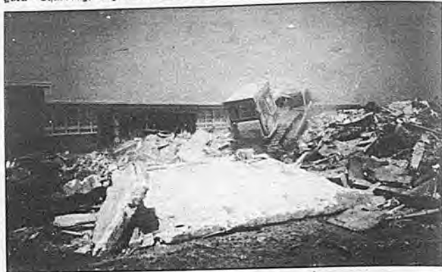
Portable classrooms were demolished at Dutch Lane Elementary School, Stewart Avenue at Levittown Parkway last week. Burns Avenue Temporaries were scheduled to be demolished this past Wednesday. The temporaries were demolished because there was no longer a need for them. They were erected in 1963 because of increased enrollment.
