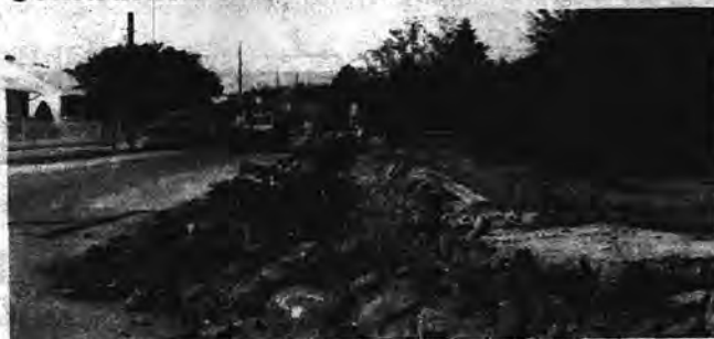
Drainage and curb work in the Northwest area of Hicksville behind Mid Island Plaza has resumed, according to Phyllis Souther, spokesperson for the Town of Oyster Bay. For the past two weeks, construction had ceased because "the private contractor of the Town of Oyster Bay, had another contract that he had to fix," Ms. Souther said. Some of the streets receiving the work are Princess Street, Nevada Street, Brighton Place, Savoy Place and Carlton Place.
