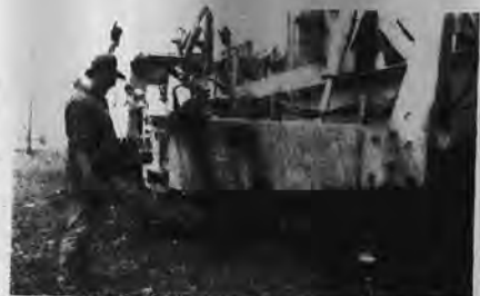
I'VE BEEN PLOWING ON THE RAILROAD. ...Workers watch as railroad plow buries power lines in track bed between Hicksville and Ronkonkoma for the LIRR main line electrification project. LILCO is providing the cable, the plow, and substation equipment modifications to accommodate the $167 million plan.
