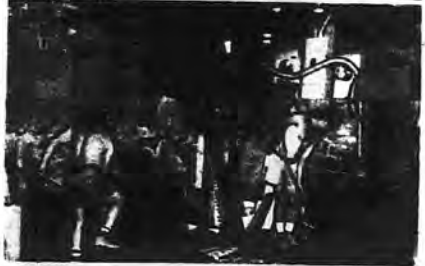
Section of original Hicksville Courthouse foundation at Heitz Place being underpinned as part of Town of Oyster Bay Community Development Project at the historic landmark. The renovation and preservation of the courthouse-jail, the home of the Hicksville Gregory Museum has Unicorn Developers, Ltd. as the general contractor. (In upper photo.)
