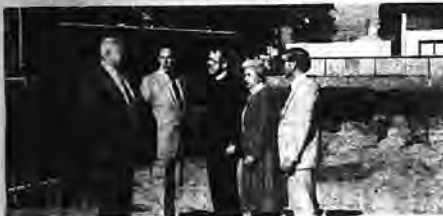
CHECKING-CONSTRUCTION PROGRESS: Oyster Bay Town Supervisor Joseph Colby (second from left) joins (from left to right) James A. Smith, Contractor, Rev. Dr. John H. Krahn, pastor of Trinity Lutheran Church and School, Oyster Bay Town Clerk Ann R. Ocker and Weldon Endorf, principal of Trinity Lutheran School, to check on the progress of the construction of the Trinity Lutheran Churches new facilities.
