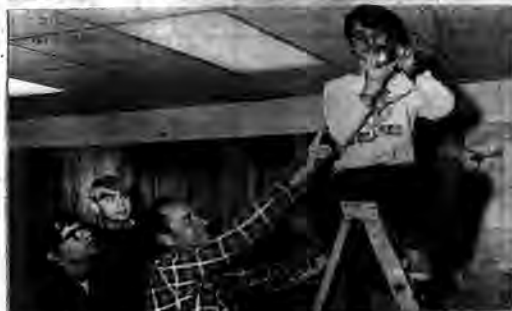
home of The Gregory Museum. Mr. Specht's excellent guidance enabled 20 temperature rise detectors and one smoke detector to be installed and wired to a central control box located in the hallway.
