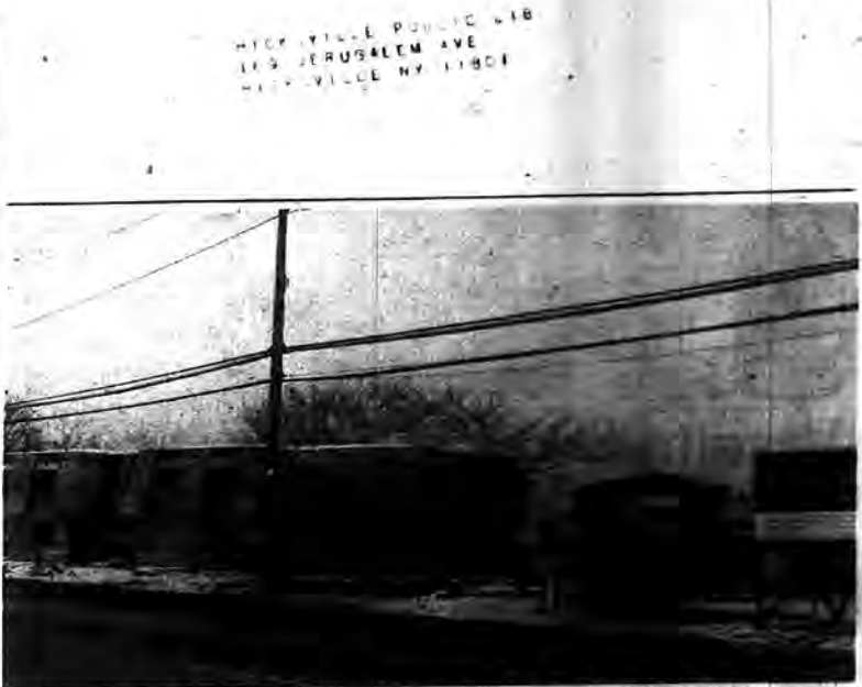
PROGRESS: Here we see the Hicksville Senior Citizens Housing Project of the Town of Oyster Bay located on Newbridge Road, Hicksville. This fine project of 72 units, will be completed in late summer, with occupancy expected in the Fall. Persons residing in the Town of Oyster Bay 62 or over will be considered, and applications may still be submitted to the Town of Oyster Bay Housing Authority, 125 West Main St., Oyster Bay, New York 11771. (Photo by Jerry Augusta)
